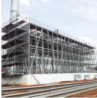
ES Power Plant
